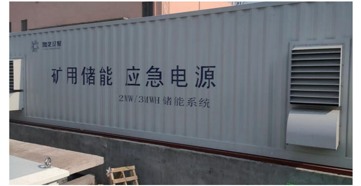
2MW/3MWh Energy Storage Emergency Power Supply for Hongqi Coal Mine
