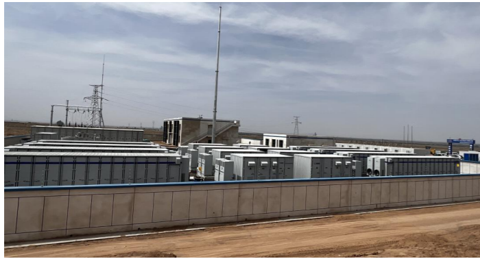
20MW/40MWh Energy Storage Power Plant
