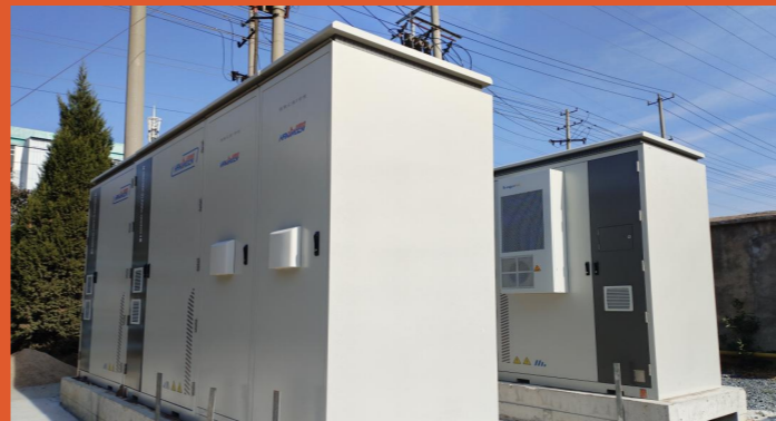
0.5MW/1MWh Use-Side Energy Storage
