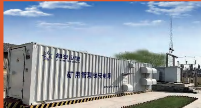
2MW/4MWh Mining Smart Security Power Supply for Henghe Coal Mine
