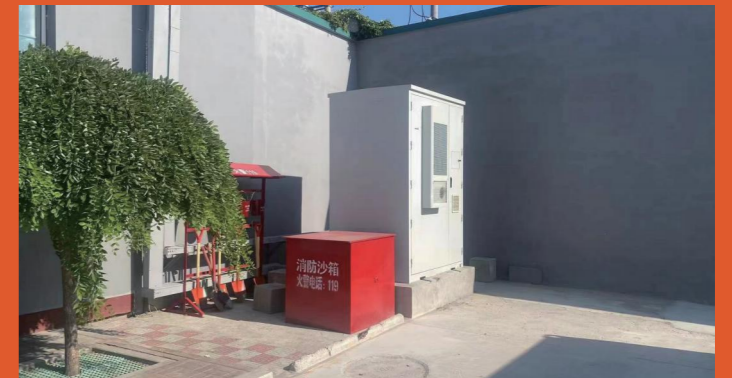
100kW/215kWh Microgrid Energy Storage Project
