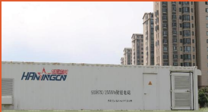
13MWh Solar Storage and Charging Integrated Project
