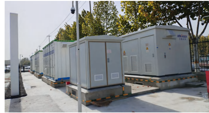
5MW/10MWh User-side Energy Storage for Hefei Haier Refrigerator Factory
